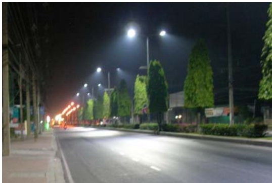
Figure 1 Test site for LED 140W road lighting for M2 class with R3 road surface
